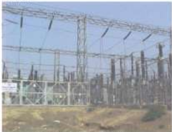
Fig. 6.1 : Tysket High Voltage Receiving Sub-station
