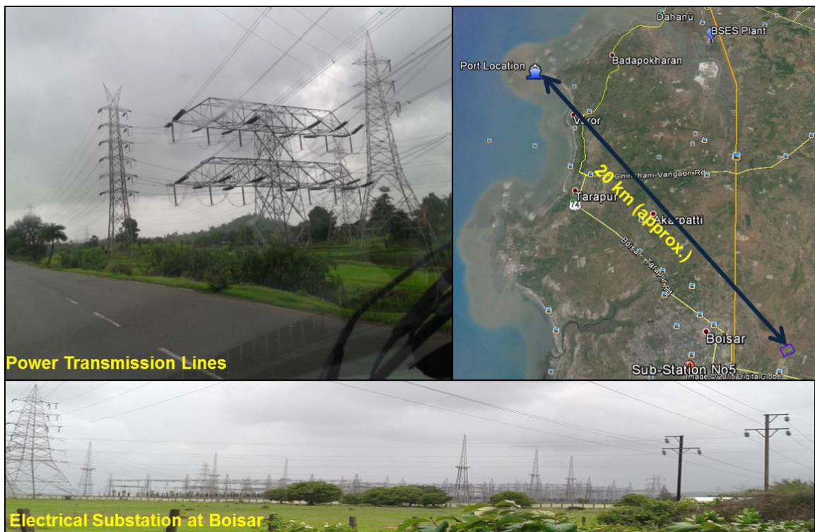
Figure 2.25 Location of Boisar Substation
